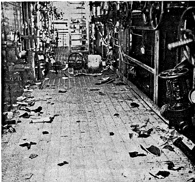
Upper level operating platform after the line rupture at DuPont's nitrogen wash unit.
